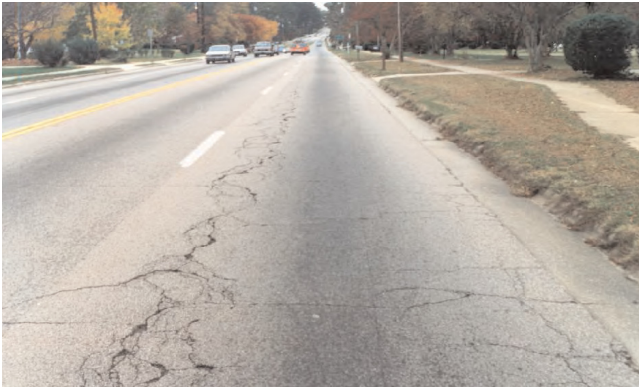
FIGURE 2 Example of severe alligator cracking.
