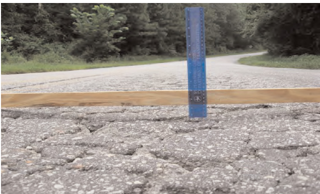
FIGURE 3 Example of severe rutting.
